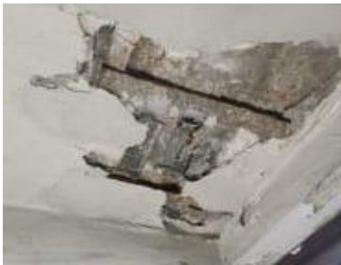
石屎剝落，鋼筋外露 Crumbling concrete revealing embedded metal support
