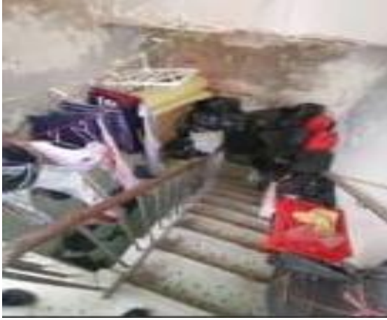
梯間雜物堆積 Clogged staircases
